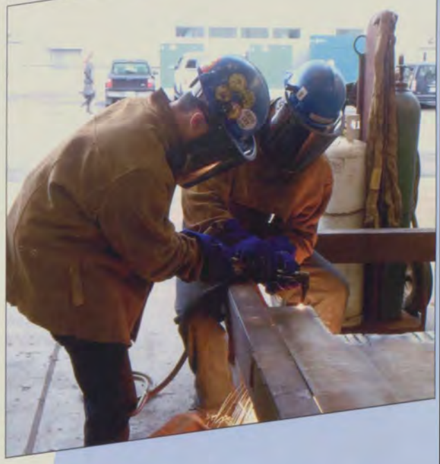
Workers show a high school students on how they cut metal. Photo | Allegra Machado
